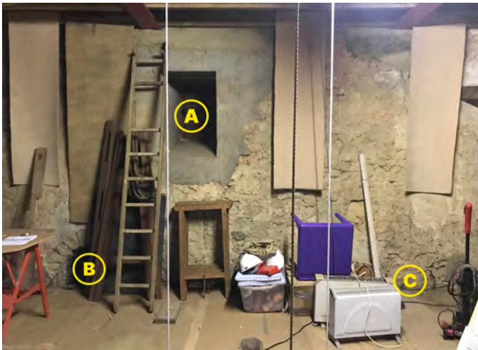
Fig 7 Bletchingley, east wall of the clock chamber, showing ? modern rectangular opening (A), reconstructed round arched aperture (B), and possible top of blocked opening (C).
