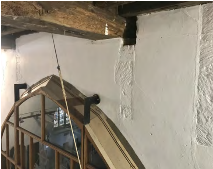
Fig 3 Bletchingley, view inside the ground floor chamber of the tower from the staircase to the middle and upper levels. Note the construction of the aperture jambs, probably formed from blocks of squared chalk sourced locally.
