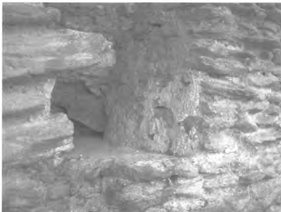
Guildford Castle: Original plaster and limewash on the side of a crenellation at the Great Tower.
